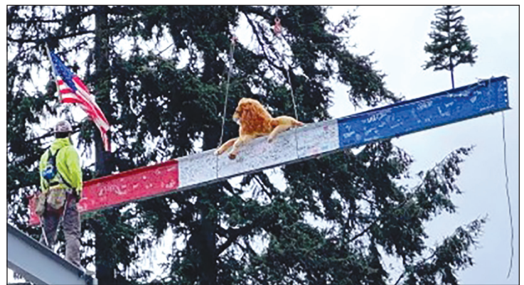
The final beam was signed by students, staff and the project team. The school's mascot came along for the ride at the topping out.
